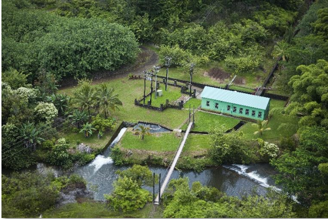
The Lower Waiahi hydro plant generates power and returns water to Waiahi stream
